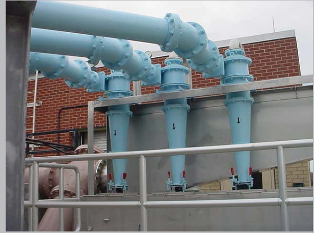
One train of ACTIFLO® Process Hydrocyclones
