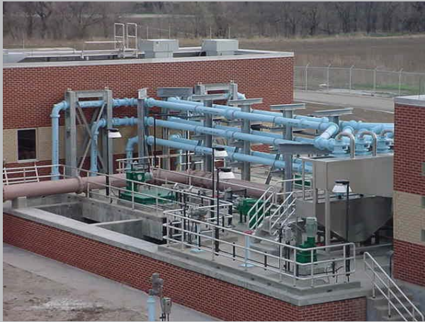
Overview of ACTIFLO® Process Basins
