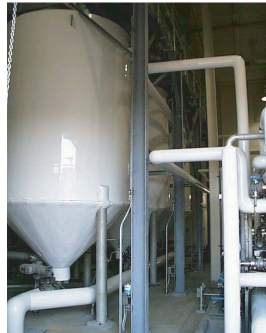
Carmel's Insulated Pasteurization Tanks
