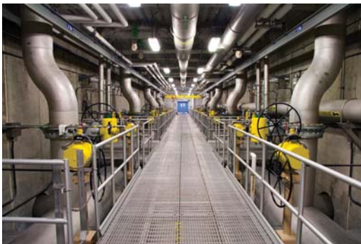
BIOSTYR Pipe Gallery Syracuse, NY
