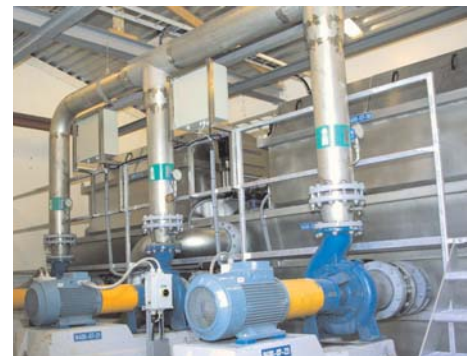
Pumps, transporting filtrated water to the cooling water system
