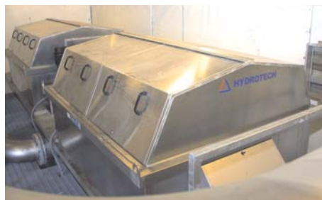
Picture showing two HDF1604-1F installed at the cooling water intake from the river
