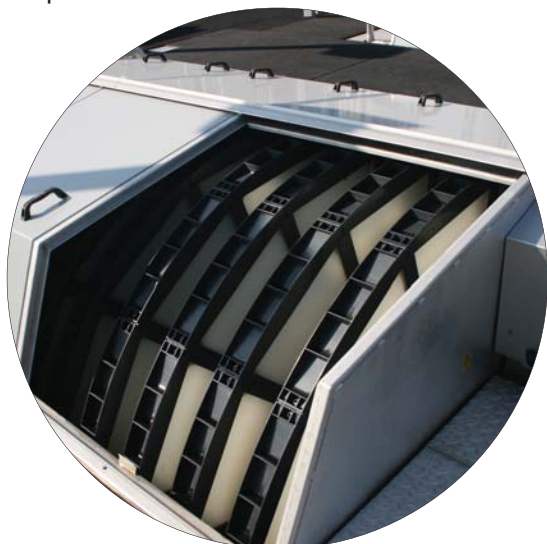
Hydrotech Discfilter Concrete Installation
